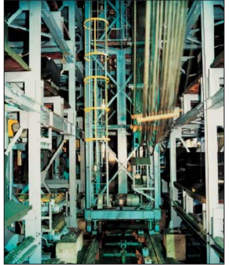
Details of the vertical moulds storage system
