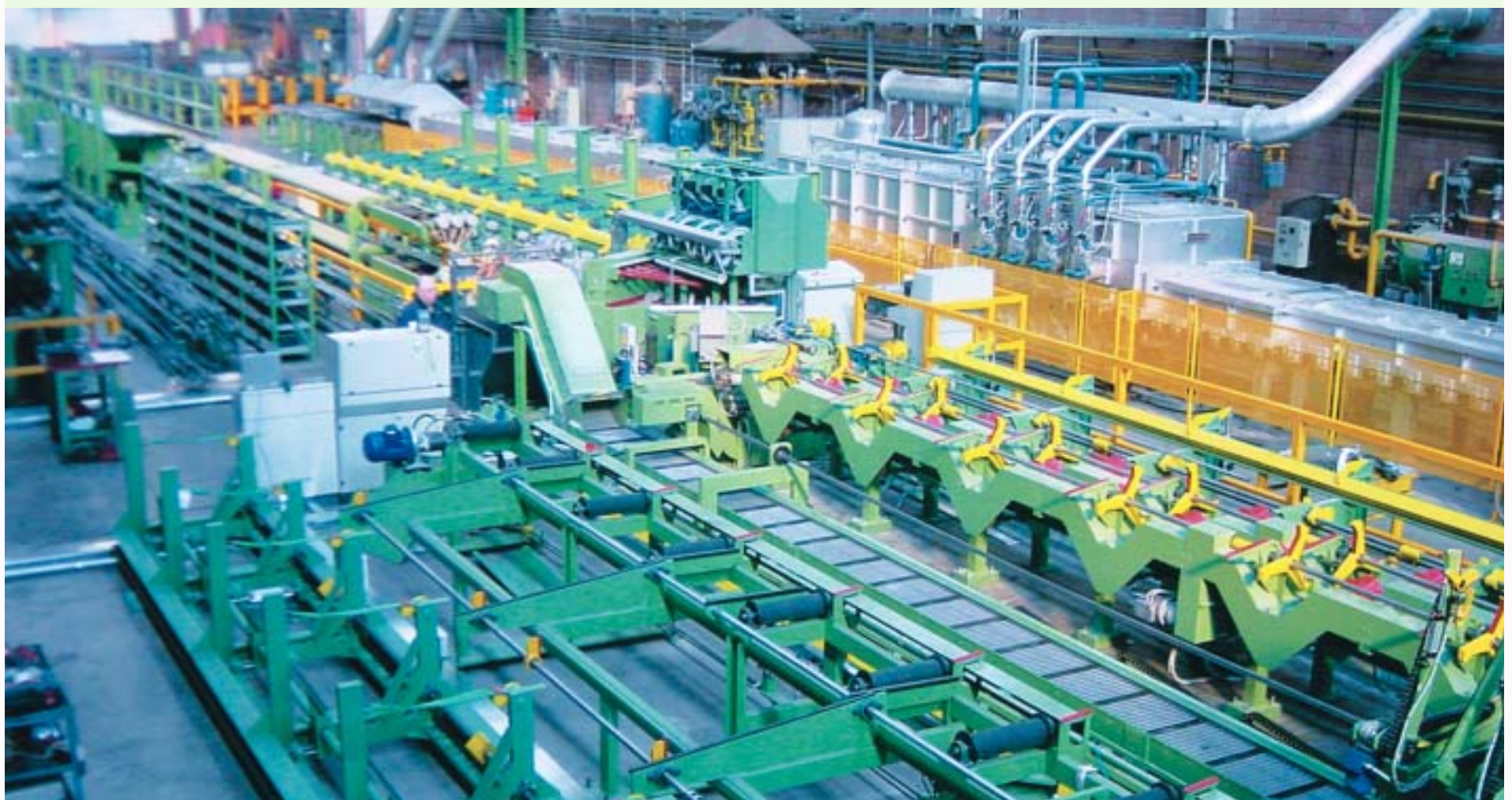
■ The installation for the handling of heat-treated tubes at Ceruti - Italy.
