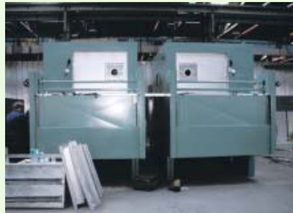
■ Gas drying tunnel
